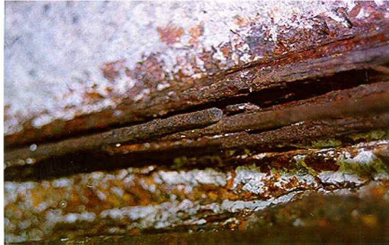
Figure 3-9 Broken wires of a corroded tendon
