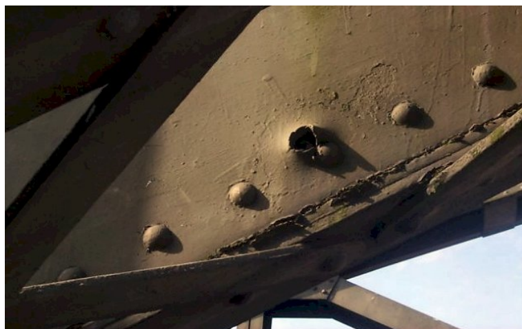
Figure 3-14 A bullet hole in a steel structure
