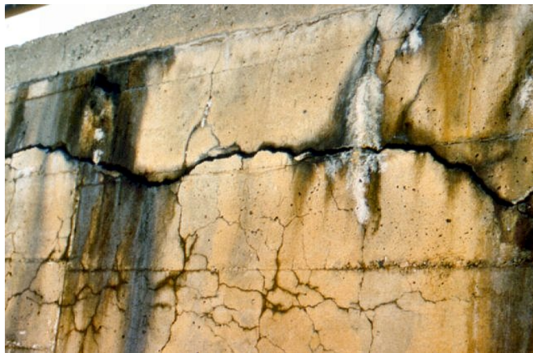
Figure 3-10 Cracking of a concrete wing wall due to ASR
