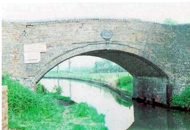
Figure 3-12 Cracking of a spandrel wall of a masonry arch bridge
