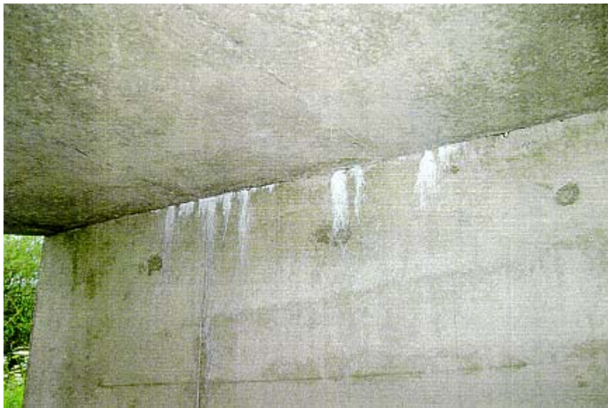
Figure 3-2 Deterioration of the construction joint between the roof and side wall of a concrete box structure due to differential movement
