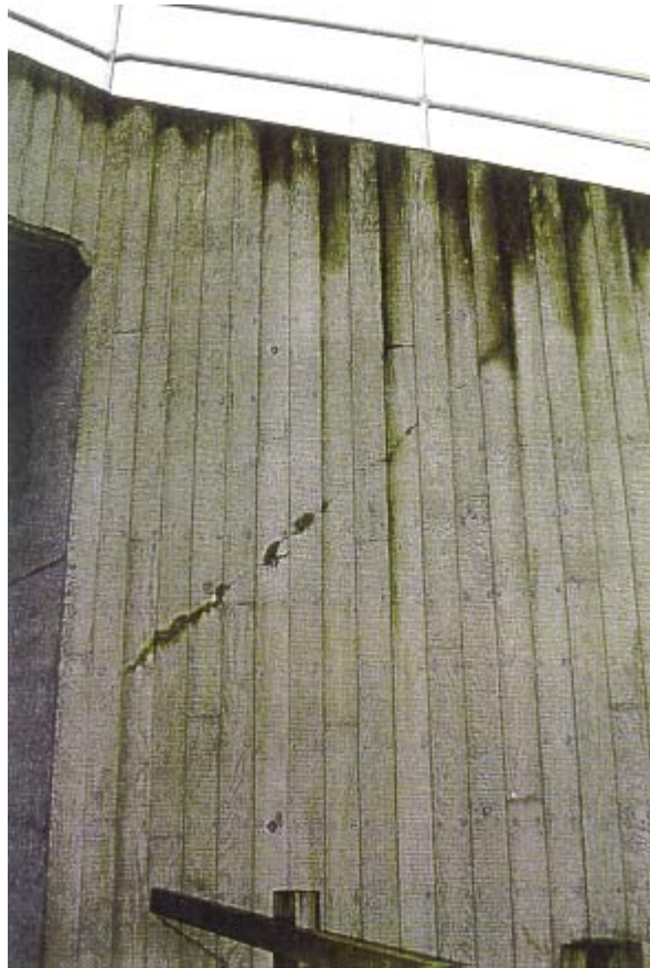
Figure 3-8 Cracking of the wing wall to a concrete box structure due to differential ground movements
