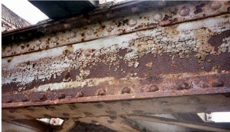
Figure 3-11 Corroded steel superstructure
