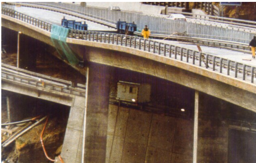
Figure 3-1 Deformation of a superstructure due to undermining of a pier by scour
