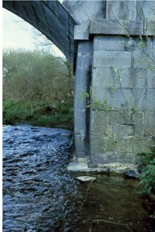
Figure 3-3 Bulging of a masonry abutment due to excessive earth pressure
