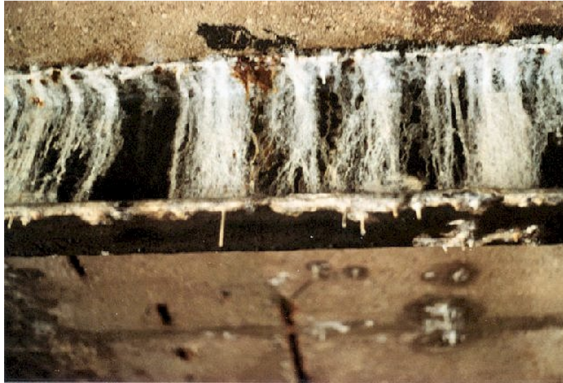
Figure 3-4 Efflorescence on steel girders due to leakage through concrete deck
