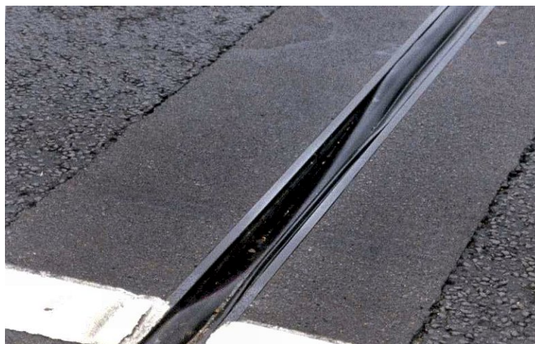
Figure 3-13 Detachment of elastomer in an expansion joint due to overstretching and/or wheel loading
