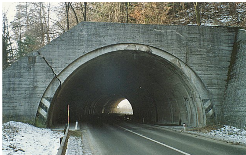
Figure 3-7 Cracking of a tunnel portal and vault due to foundation instability
