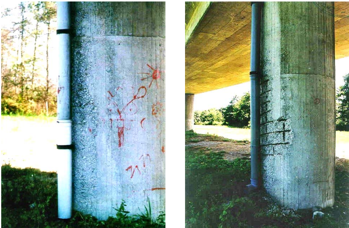
Figure 6-2 Condition of a column in 1997 and 2000
