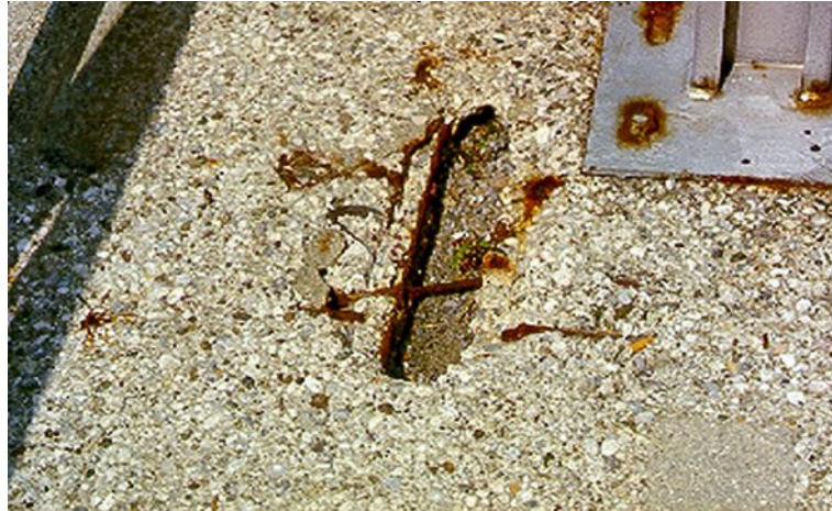
Figure 3-5 Freeze-thaw damage of a footway aggravated by the action of de-icing salts
