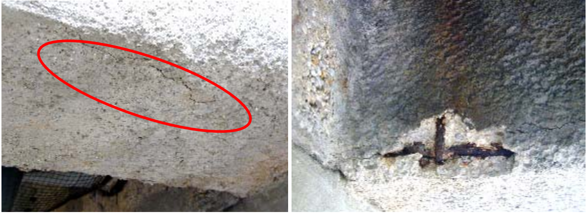
Figure D.5: Cracks in girder D (left) and corroded reinforcement (right)
