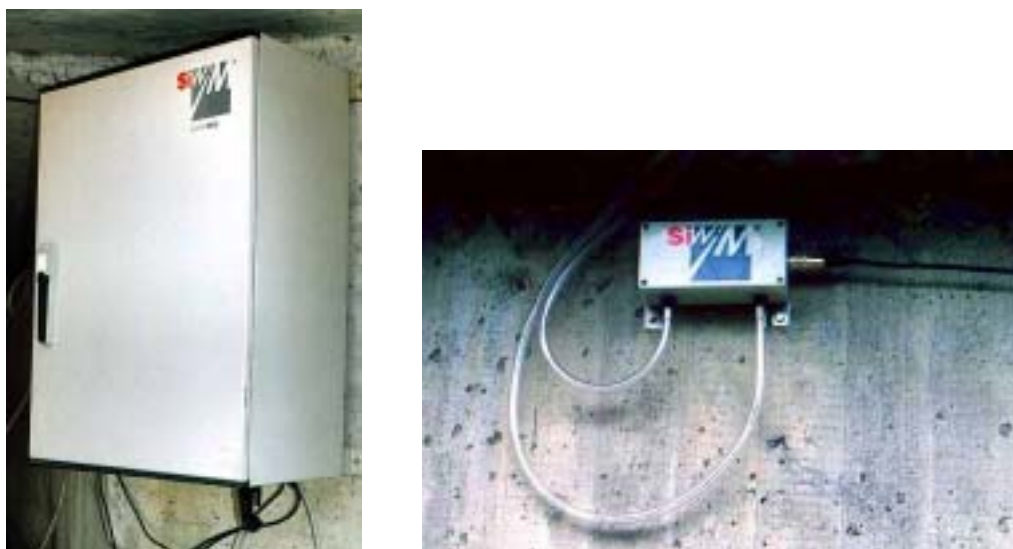
Figure D.9: Data acquisition unit (left) and pneumatic converter (right)
